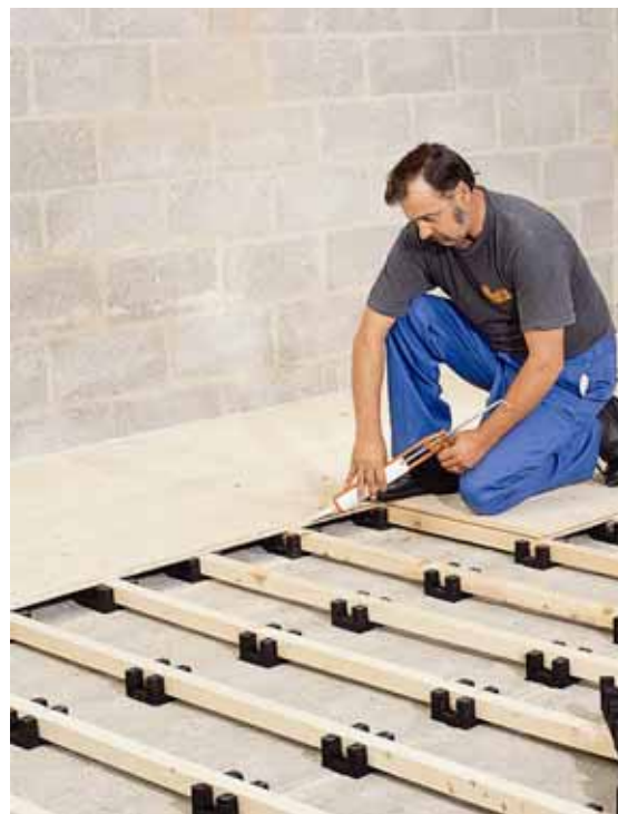
Plywood decking fixed to battens suspended on rubber pads to conform to the force reduction and deformation limits of an area elastic or combined elastic floor to BSEN 14904
