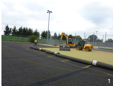
Carpet being carefully rolled up using the bucket of an excavator. The excavator is positioned on the carpet to avoid damaging the shockpad
