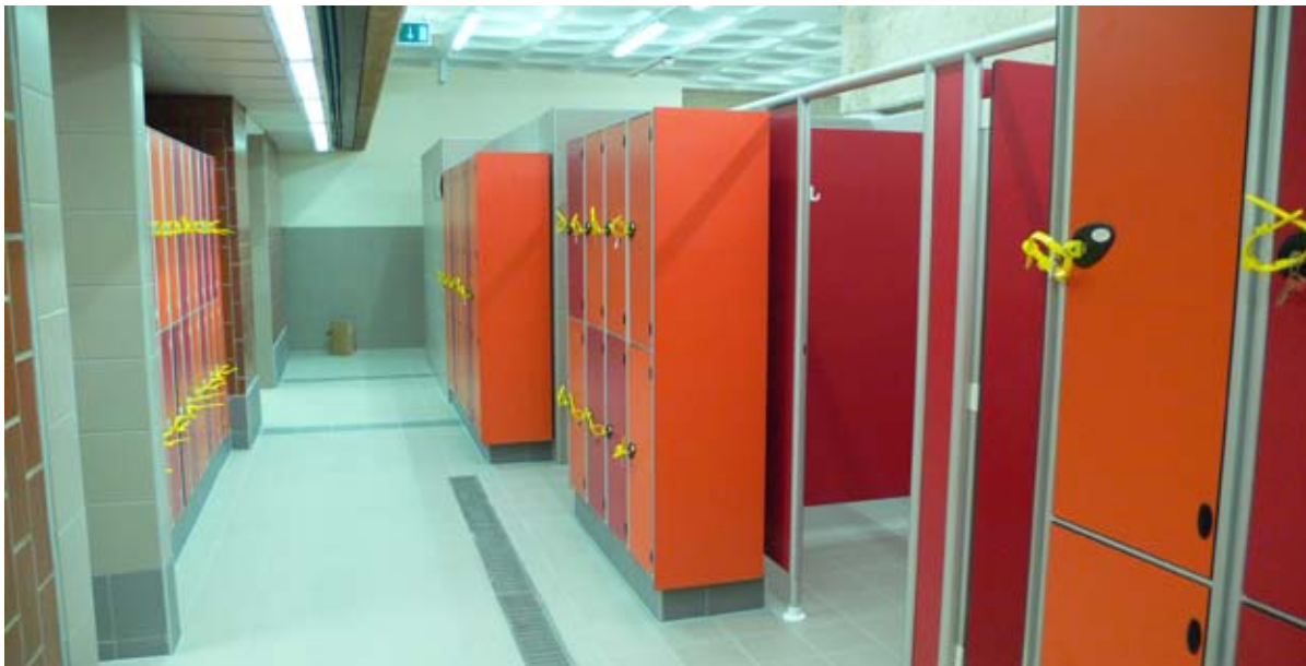
New slip resistant tile floor, lockers and accessible cubicles to upgrade a 1980's changing area
